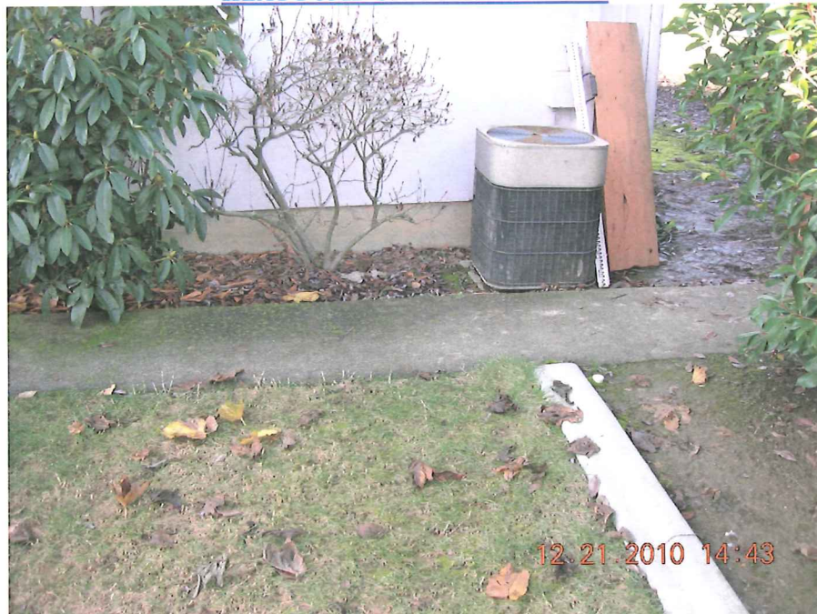
HEAT PUMP ON CONCRETE PAD
