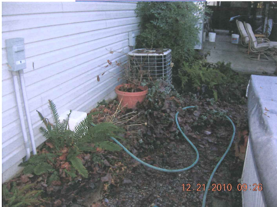
HEAT PUMP ON CONCRETE PAD
