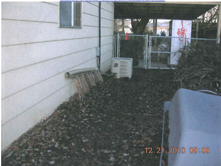
HEAT PUMP ON CONCRETE PAD
