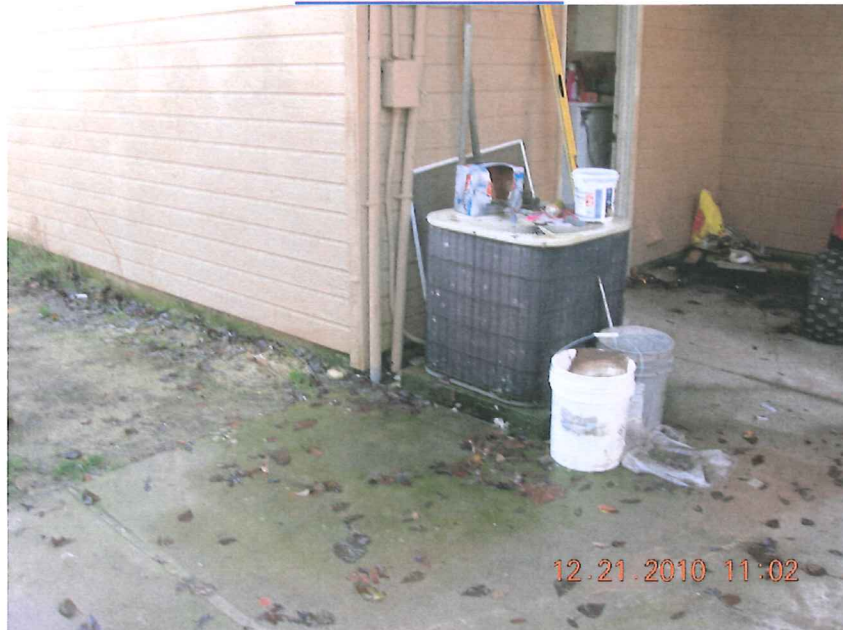
HEAT PUMP ON PAD
