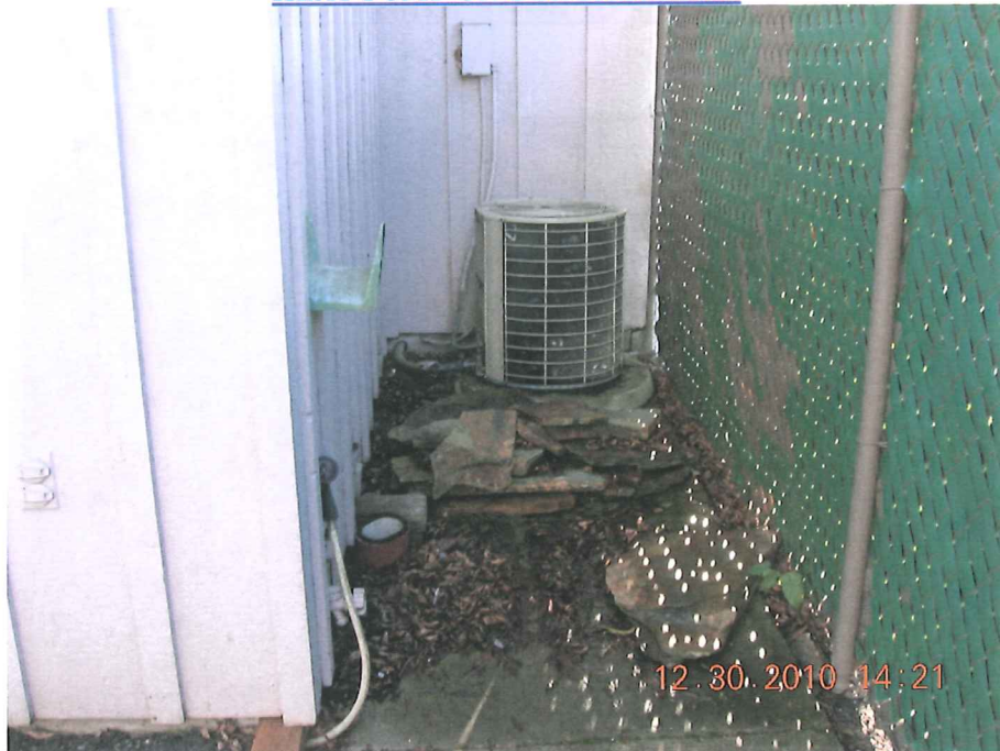
HEAT PUMP ON CONCRETE PAD
