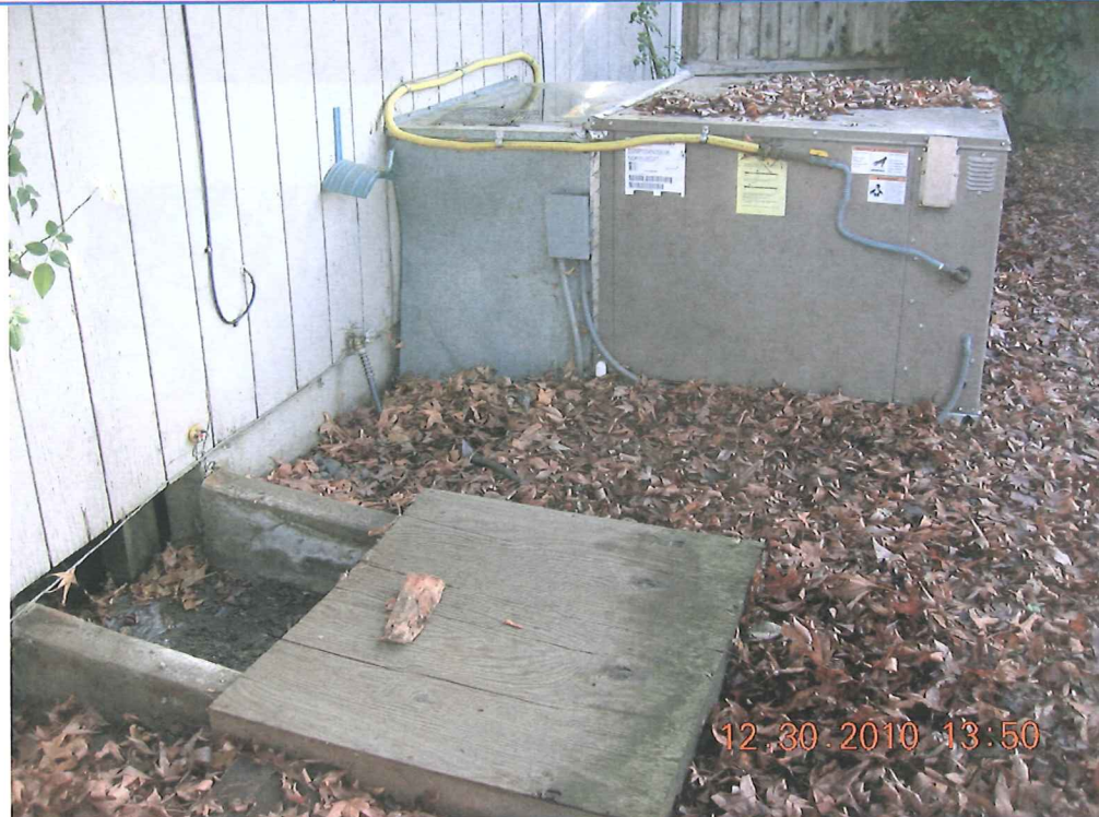
CRAWL SPACE ACCESS (TO THE LEFT) AND A HEAT PUMP ON CONCRETE PAD
