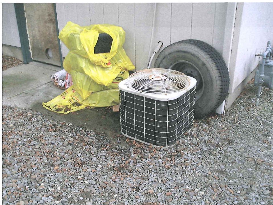
HEAT PUMP ON CONCRETE PAD
