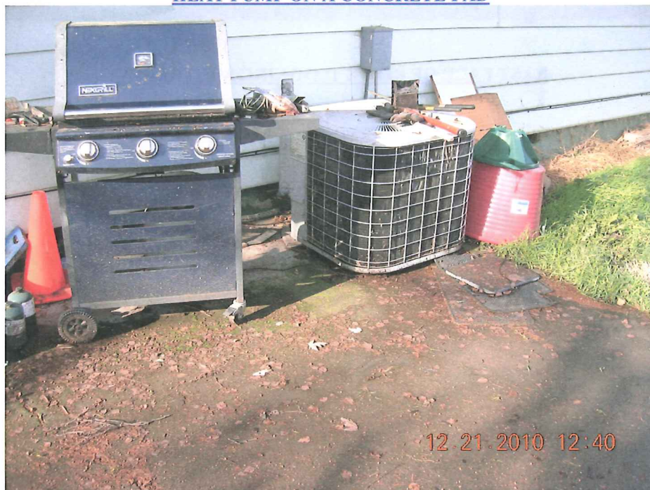
HEAT PUMP ON A CONCRETE PAD
