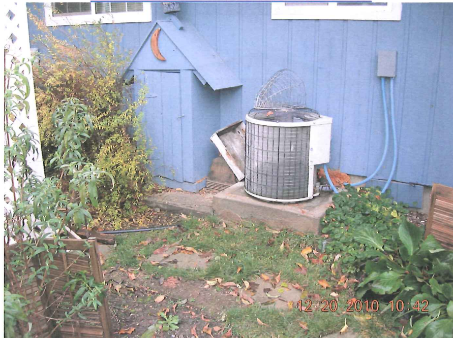
HEAT PUMP ON CONCRETE FOUNDATION
