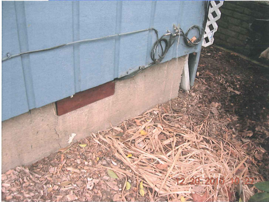
TYPICAL FOUNDATION VENT (ALL COVERED)
