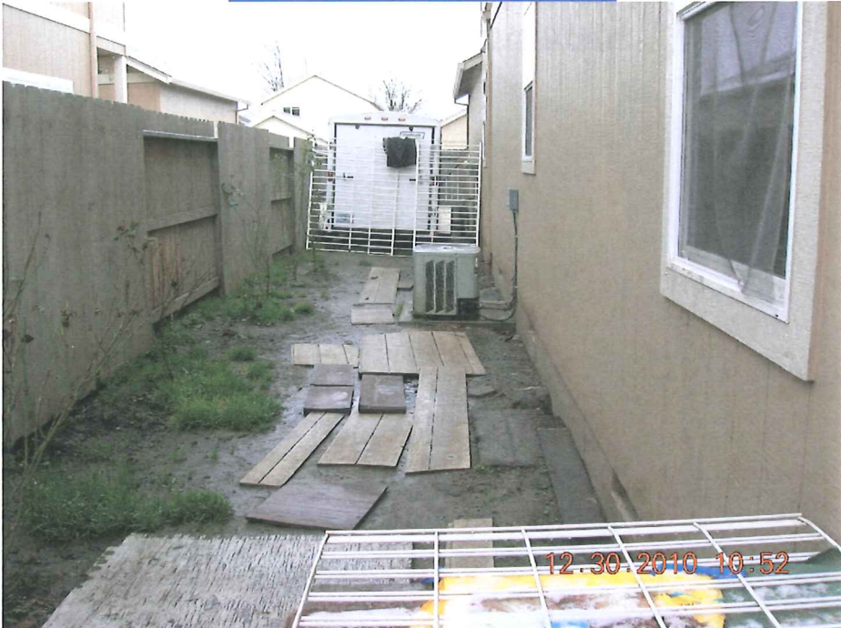
HEAT PUMP ON CONCRETE PAD
