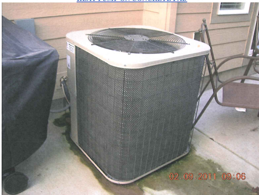
HEAT PUMP ON CONCRETE PAD
