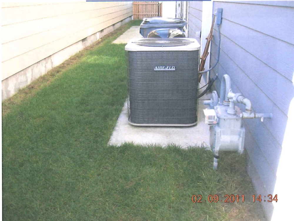
HEAT PUMP ON CONCRETE PAD
