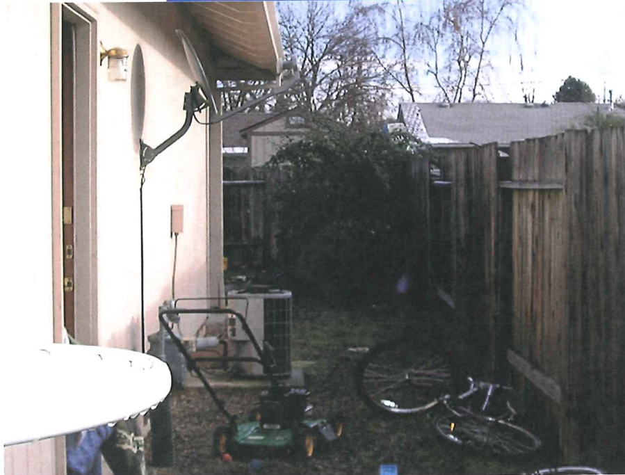
HEAT PUMP ON CONCRETE PAD
