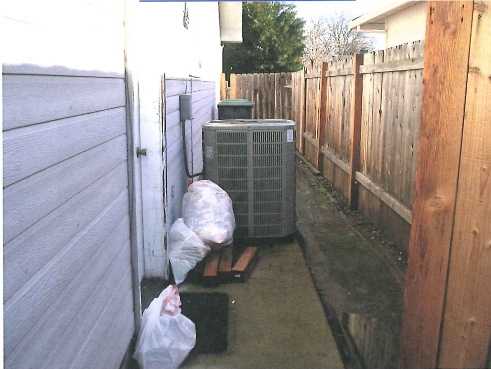
HEAT PUMP ON CONCRETE PAD
