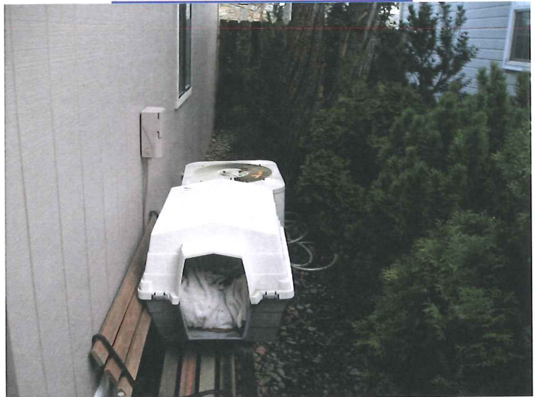
HEAT PUMP ON CONCRETE PAD
