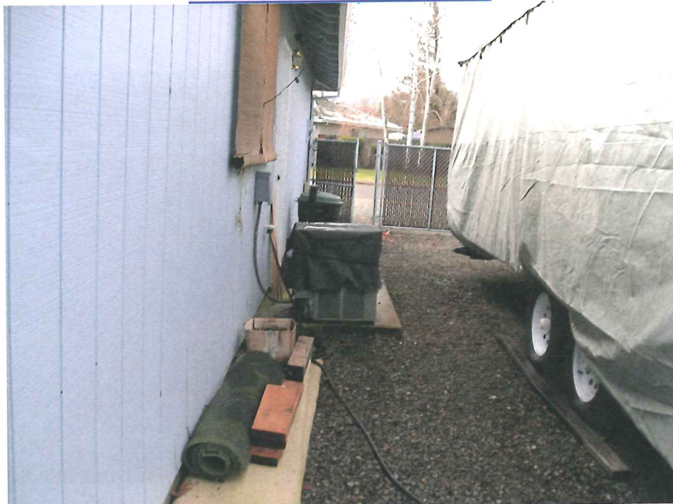
HEAT PUMP ON CONCRETE PAD
