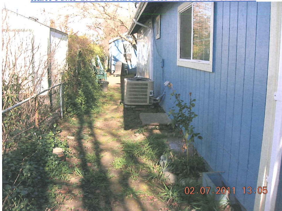
HEAT PUMP ON CONCRETE PAD AT WEST FACE OF HOME
