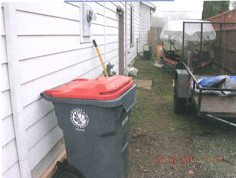
HEAT PUMP ON CONCRETE PAD
