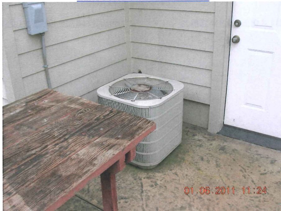
HEAT PUMP ON CONCRETE PAD
