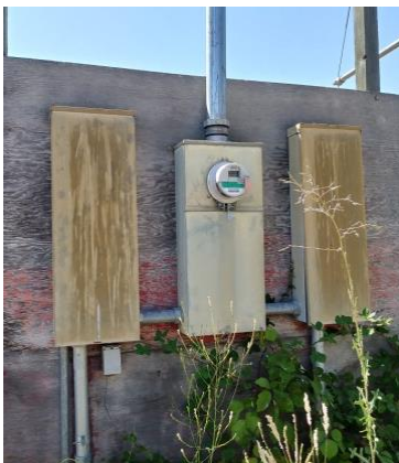
Exterior meter on site.
