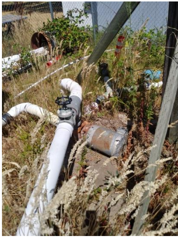
Pump outside storage building.
