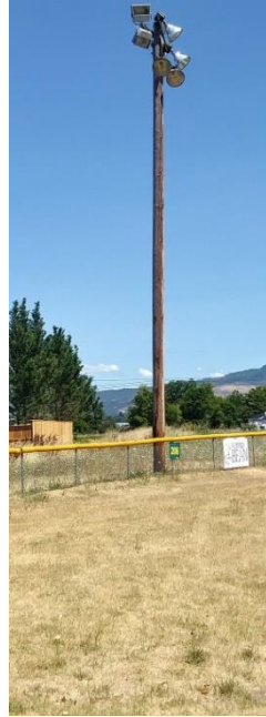
Utility pole with field light.
