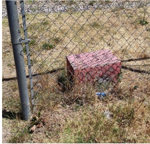
Water valve located at each field.
