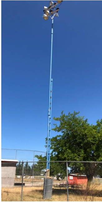
Steel pole with field light and exposed concrete pier foundation.
