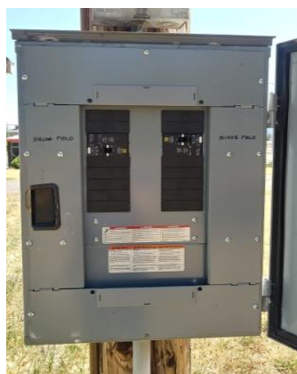
Field light exterior circuit breaker.
