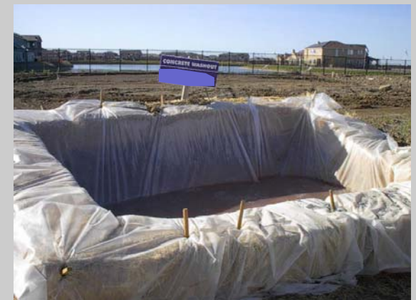
An example of a properly designed concrete washout. Washouts can be scaled down for use on smaller projects.
