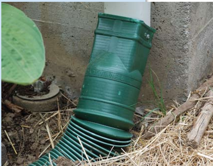
Figure 14. Downspout connected to downspout extension that directs flow away from a building's foundation. Note sheet-metal screws.
