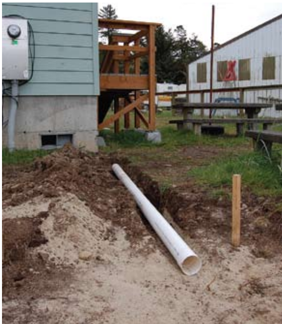
Figure 22: Four-inch ABS pipes here will convey water from this building into a rain garden. Pipes like these must be graded to drop about 1 inch for every 10 feet so water flows away from the building but does not build up too much velocity by the time it arrives in the rain garden. (Photo: Robert Emanuel, OSU)
